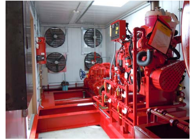
Diesel Vertical Turbine Fire Pumps
