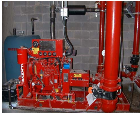
Diesel Horizontal split Case Fire Pumps
